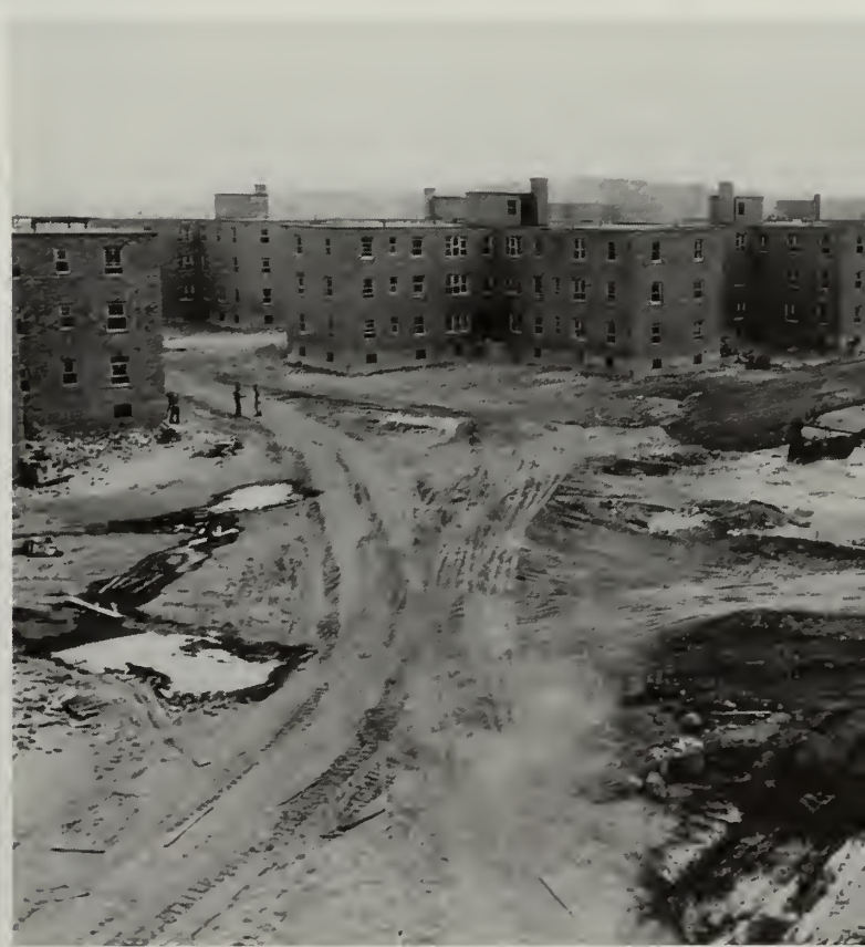
Columbia Point under construction, in a series of 1953 photographs. Boston Housing Authority.
